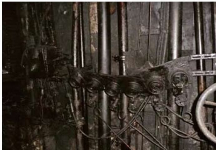
^The result of an engine room fire
