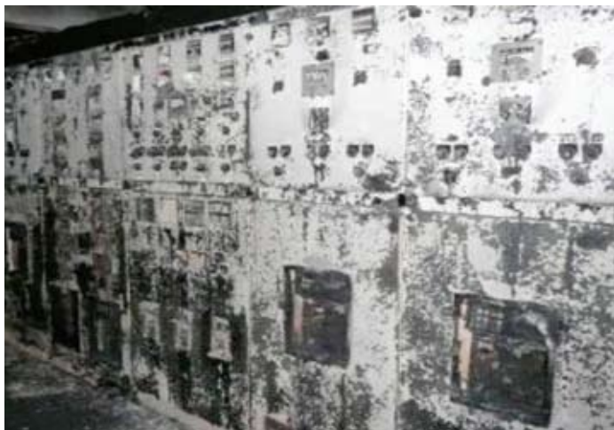
^Switchboard after an engine room fire
