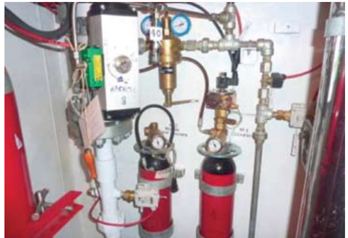
^CO 2 release systems can be complex. Have clear signage
