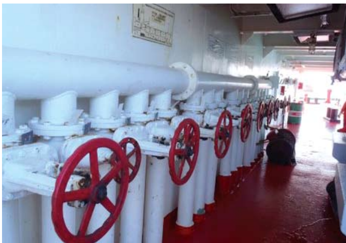
^Sprinkler valves on the main deck. No instruction or identifying stencils
