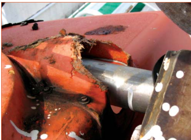
DAMAGED EQUIPMENT IN SERVICE
