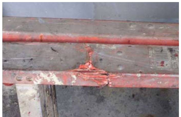
^ A portable ladder with visible signs of damage. This ladder should not be used
