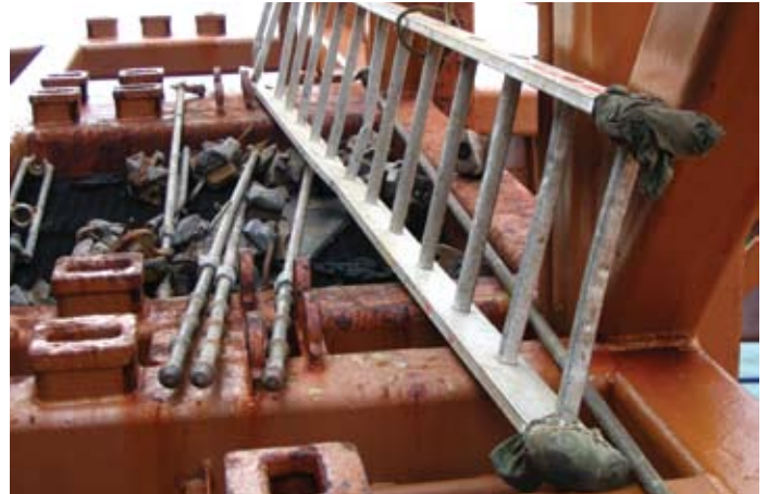
^ A severely damaged portable ladder beyond repair. This ladder should not be used
