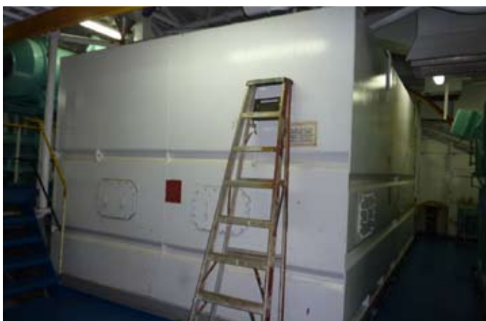
^ Portable stepladder kept in the engine room showing signs of rusting, not stowed on a rack or kept away from heat sources
