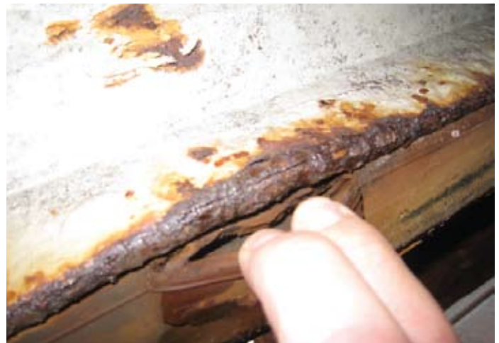
^ Damaged packing rubber seals
