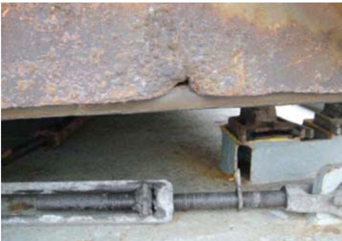
^ Damaged hatch cover edges would allow water ingress – sufficient to cause water damage to water-sensitive cargo
