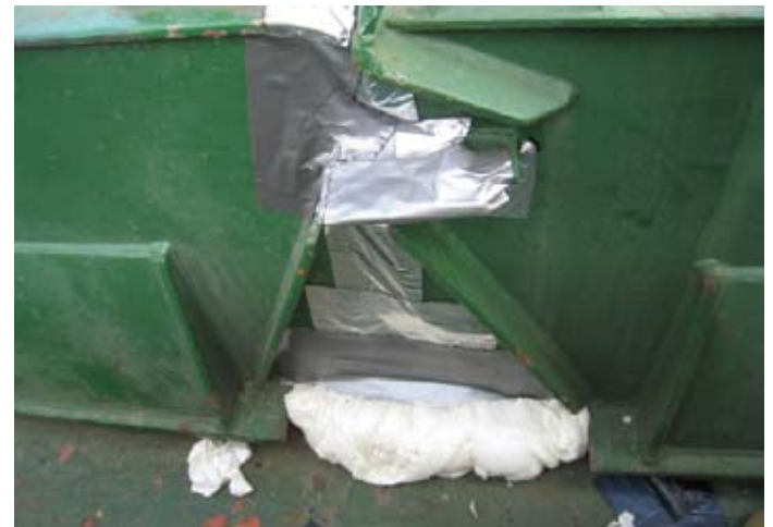
^ The use of foam and tape is not a primary means of preventing water ingress
