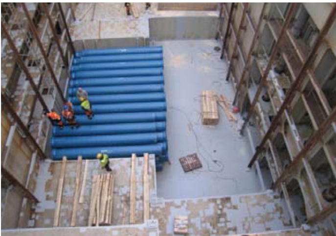
^ Pipes stowed correctly
