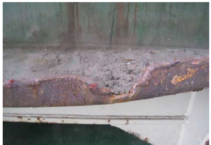
^ Damaged channel bars – potentially allowing water ingress
