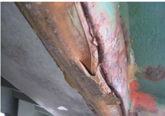
^ Damaged packing channels and seals – sufficient to allow water ingress
