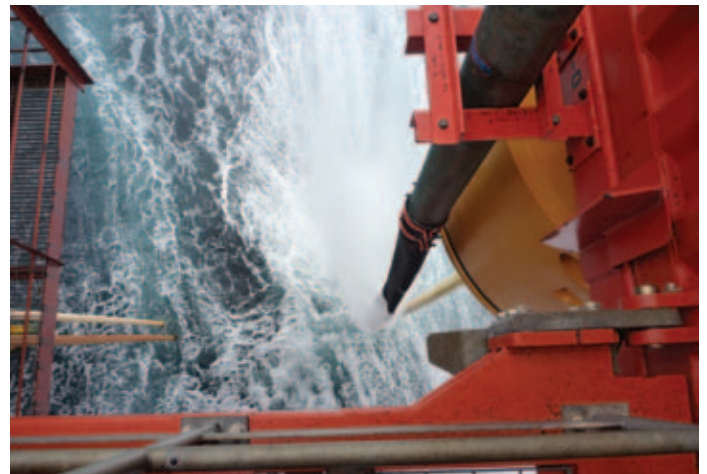
^ Water discharge from production unit
