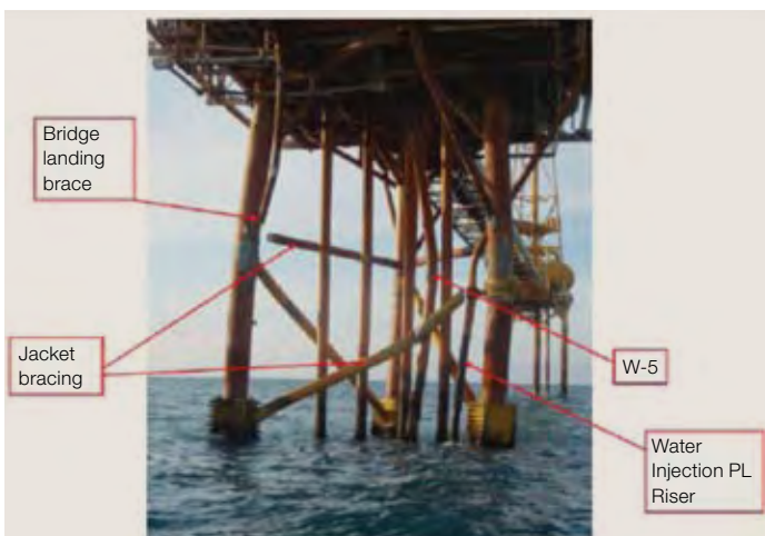
Damage to Ekofisk 2/4's load-bearing structure, conductor and riser (source: ConocoPhillips)
