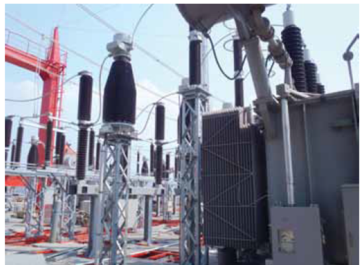
^ High voltage installation on special power station ship
