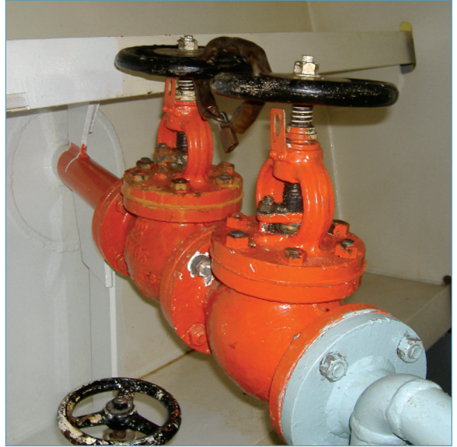
OILY WATER SEPARATOR OVERBOARD LINE
