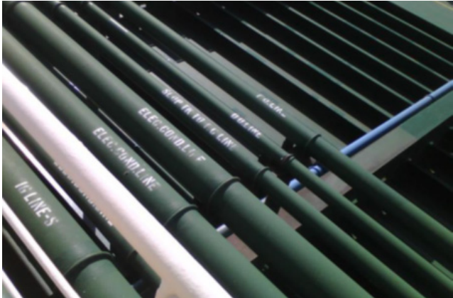
Figure 5: Typical inert gas piping
