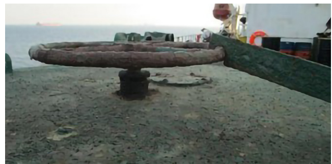
Figure 13: Typical pitting corrosion
