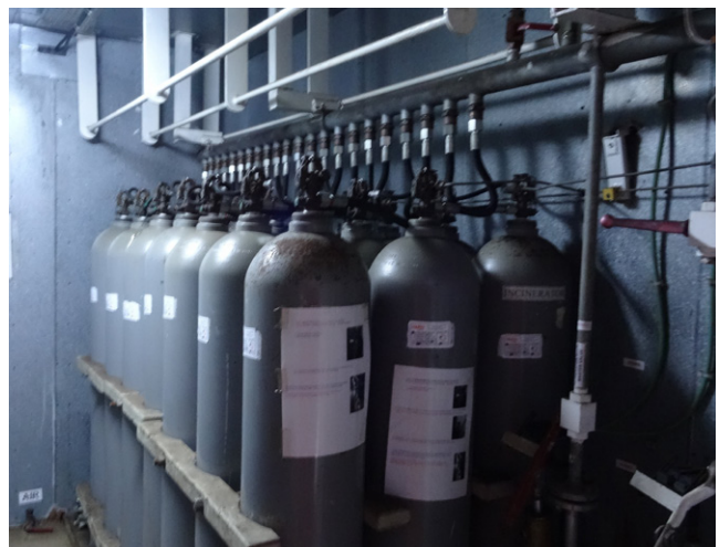
Figure 6: Typical CO 2 piping
