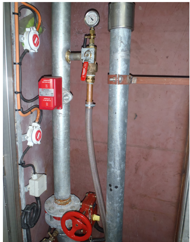
Figure 4: Typical sprinkler system piping
