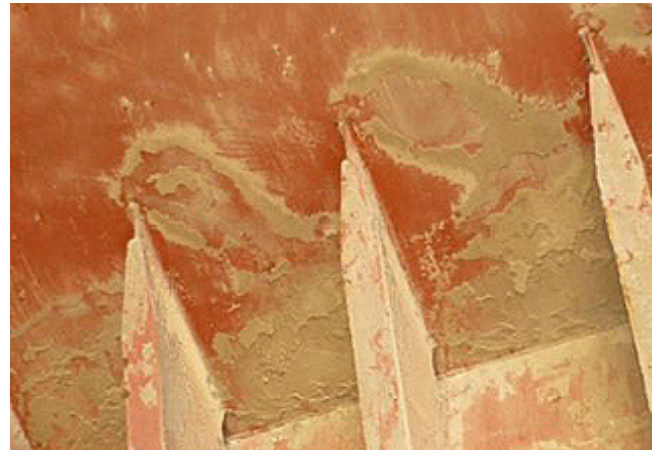
Figure 7: Cement residues in less accessible parts of the hold
