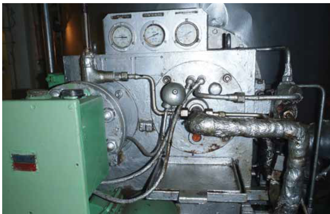
^ Always follow manufacturer's advice with boiler burners
