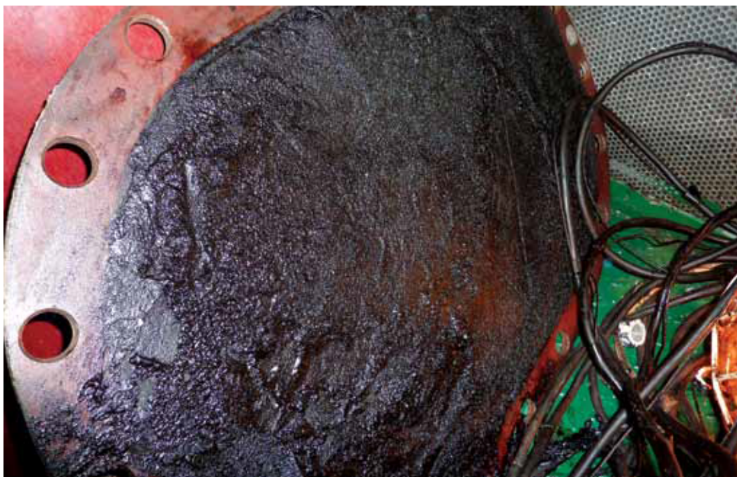
^ Fuel oil service tank manhole cover showing contamination of fuel
