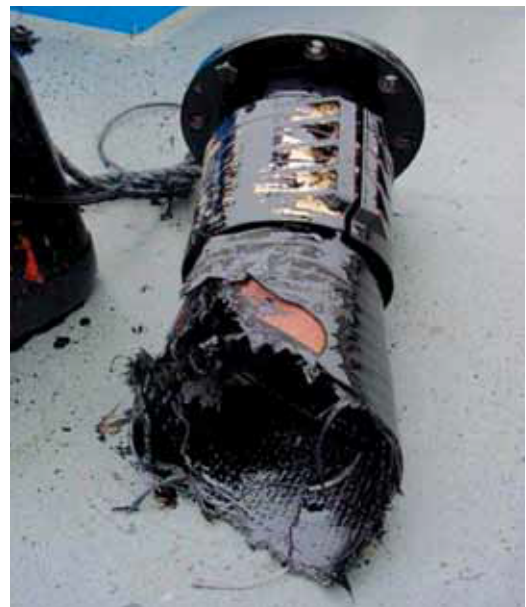
^ Failed bunker hose
