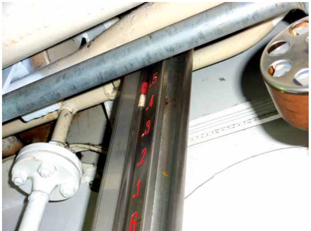
^ Bunker tank level indication
