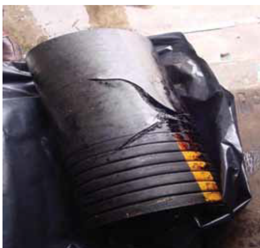
^ Cropped section of damaged bunker hose
